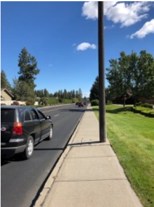
Figure 2: Encroachment on sidewalk of utility pole.
