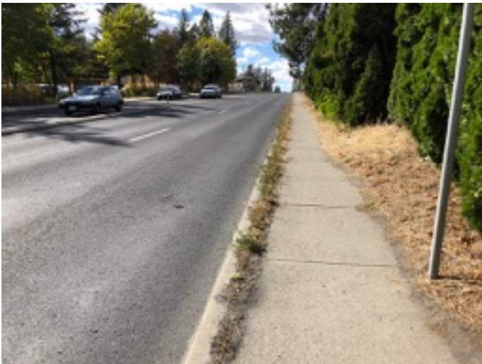
Figure 7: Vegetation and poor condition of sidewalk.
