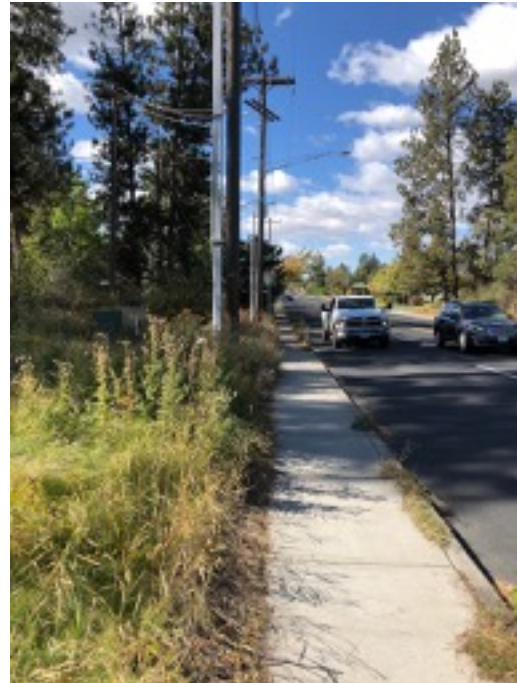
Figure 3: Vegetation encroaching on sidewalk.
