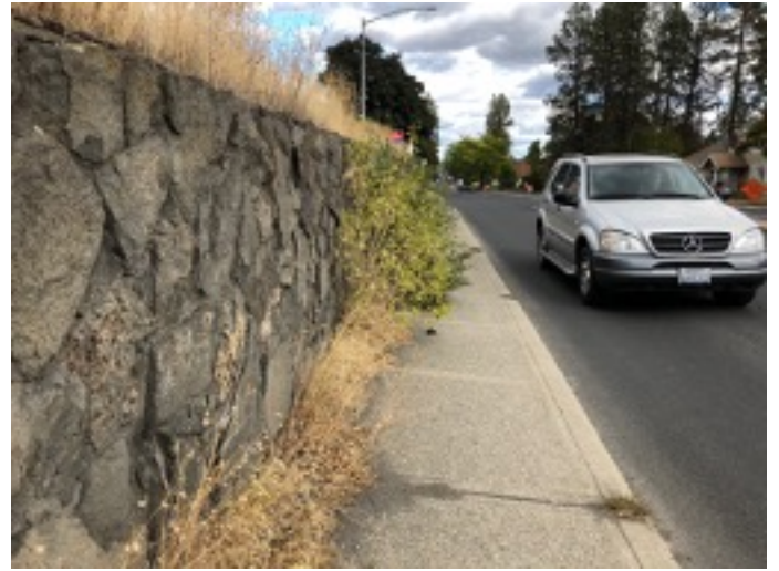
Figure 8: More vegetation encroaching on sidewalk, making the pathway very narrow for pedestrians.
