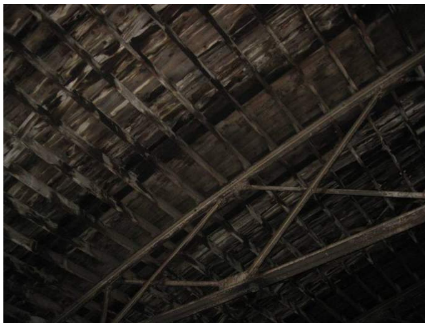
Photo 10: Typical North Area Roof Moisture Damage
