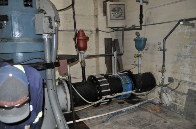
Pump 1 and Piping
