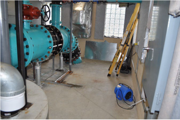
Well 1 Piping in Building
