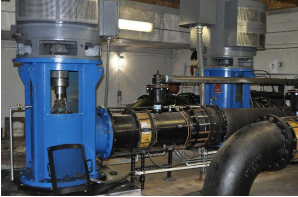
Nevada Pumps and Piping
