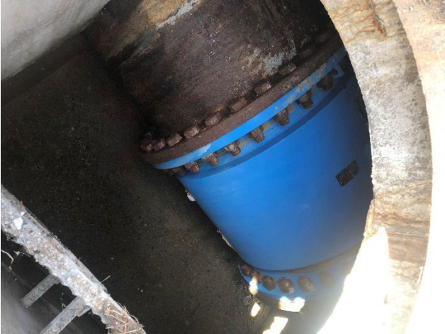
North Hill Pressure Zone Flow Meter Vault
