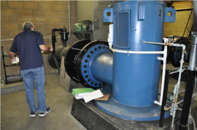
Pump and Pipe Discharge
