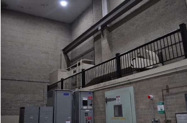
Chlorine Room and HVAC
