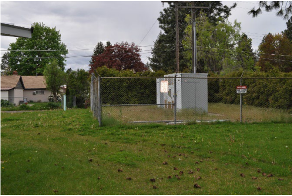
Fenced Power Area
