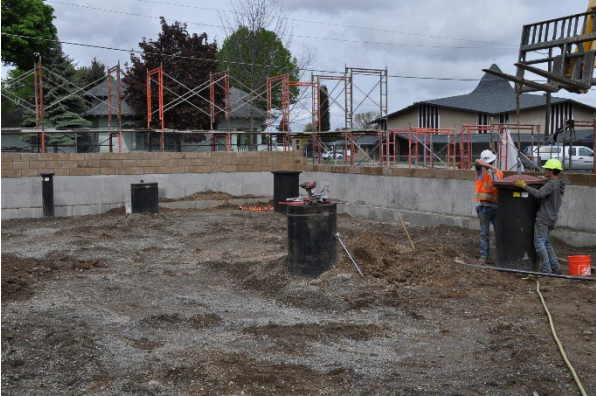
Well Station A
