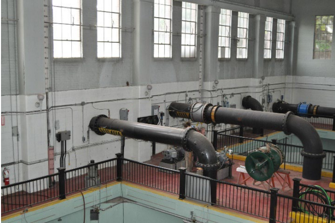
Pumps 3-6 Discharge Piping
