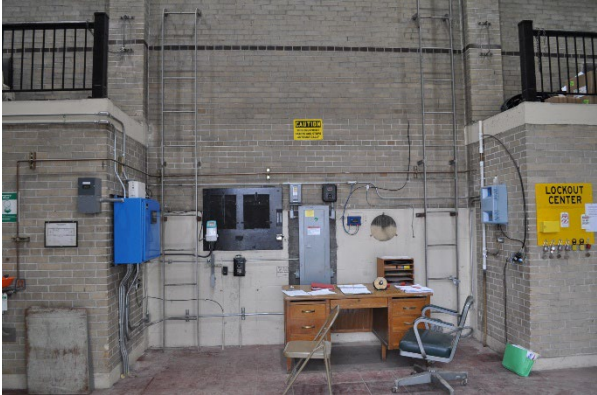
Chlorine Analyzer Area
