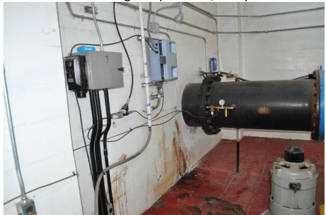
Monitoring Sample Point, Pump 1
