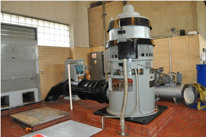
Pump and Discharge Piping
