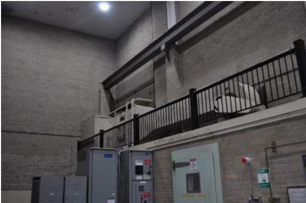
Chlorine Room and HVAC
