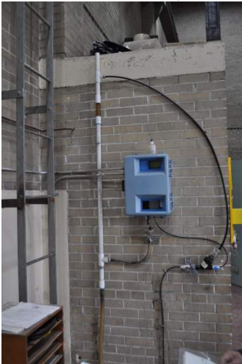
Hoffman Chlorine Analyzer
