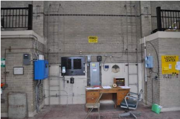
Chlorine Analyzer Area
