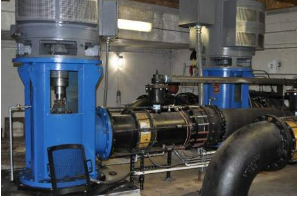
Nevada Pumps and Piping
