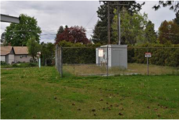
Fenced Power Area
