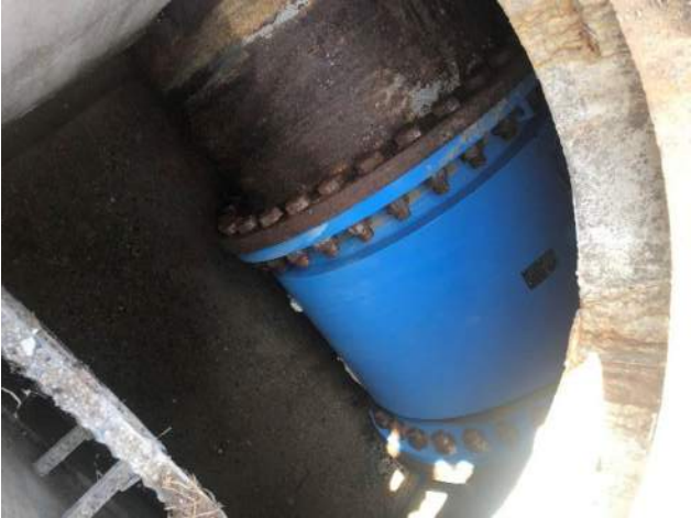
North Hill Pressure Zone Flow Meter Vault
