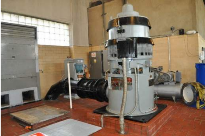
Pump and Discharge Piping
