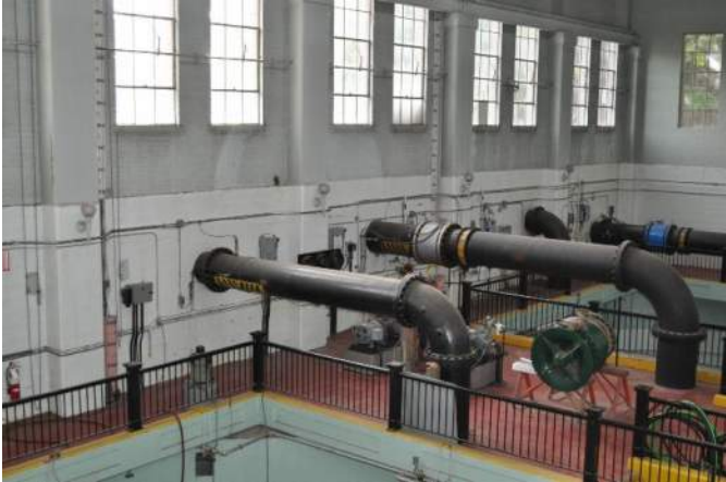
Pumps 3-6 Discharge Piping
