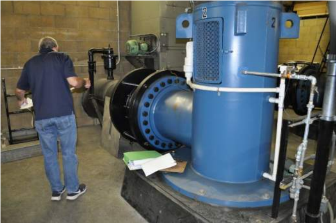
Pump and Pipe Discharge
