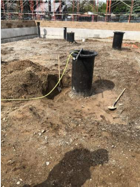
Example Well Casing
