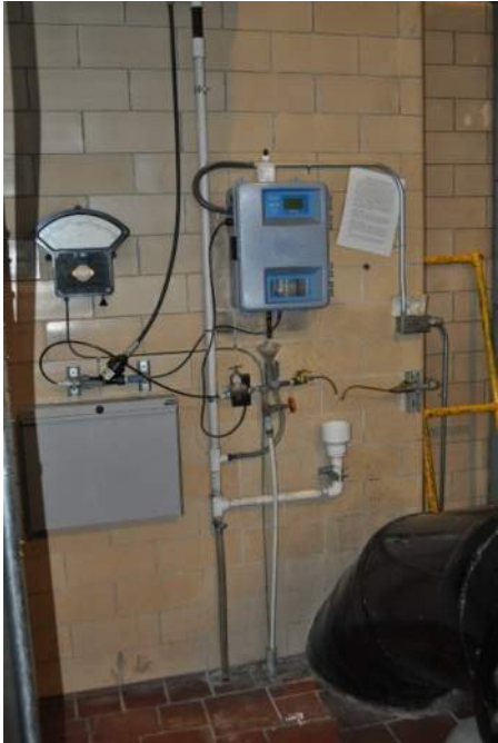
Parkwater Chlorine Monitor
