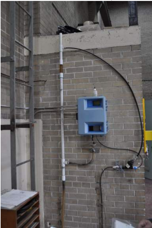
Hoffman Chlorine Analyzer
