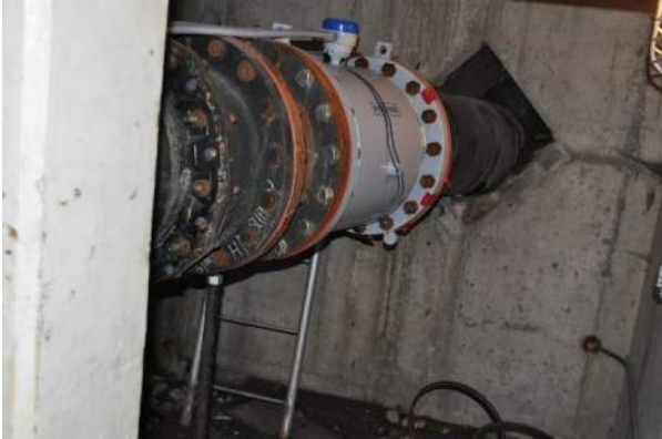
Nevada Flow Meter Tunnel
