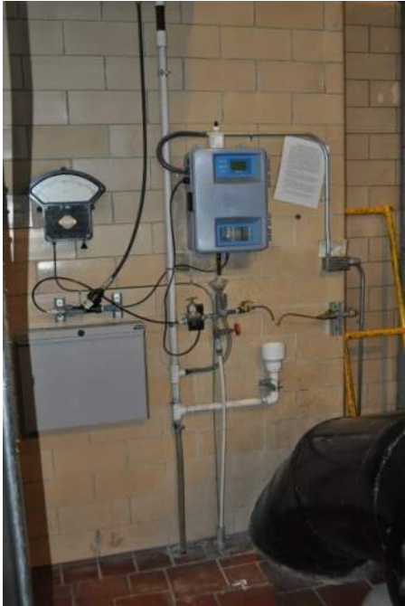
Parkwater Chlorine Monitor
