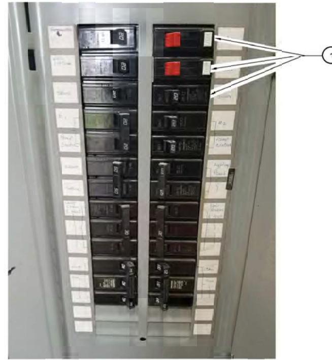
STATION SERVICE PANEL PHOTO
