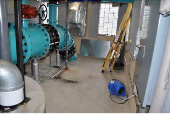
Well 1 Piping in Building
