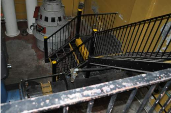
Future Pump Space
