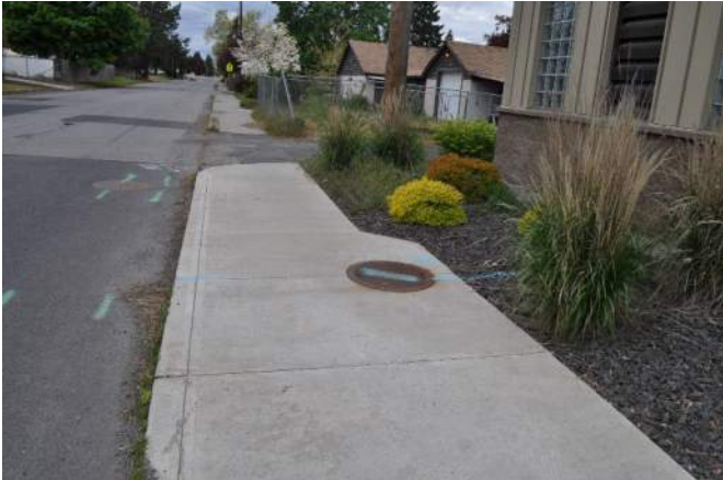
Well 1 Meter Vault
