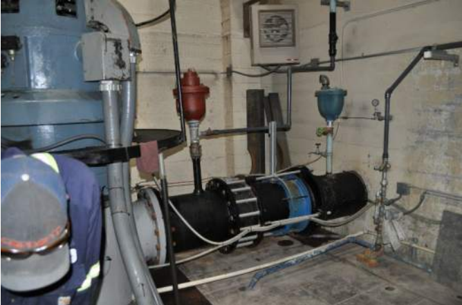
Pump 1 and Piping
