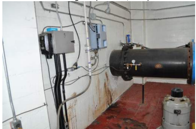
Monitoring Sample Point, Pump 1
