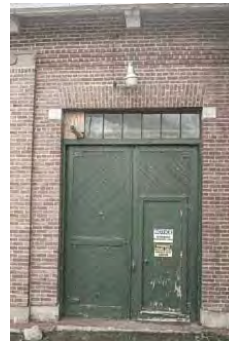
Well Electric Entry Door Looking SW.jpg
