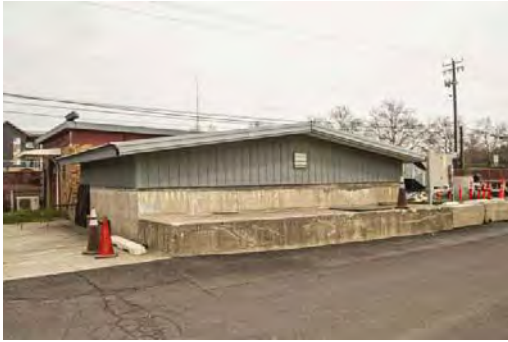
Nevada Street Well House Looking North.jpg
