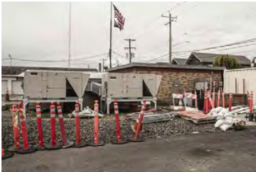
Nevada Street Well and Control Room Looking West.jpg
