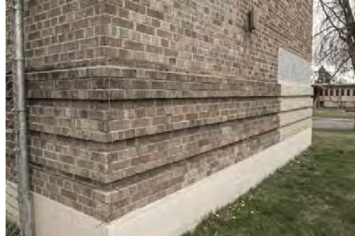
Hoffman Well Close View of Water Table Looking SE.jpg
