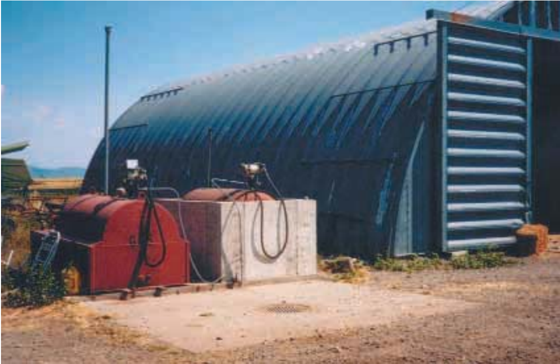
Figure 31 Left hand tank is a double walled tank
