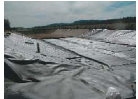
Figure 5 High Density Polyethylene Liner
