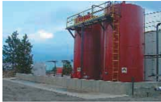
Figure 2 Solid Pour Concrete Secondary Containment
