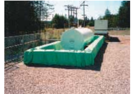
Figure 33 Temporary Containment unit (made of large concrete blocks and liner)
