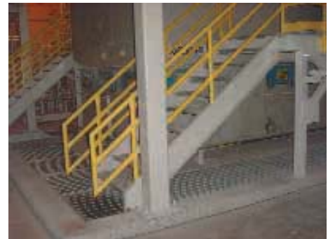
Figure 4 Example of a secondary containment area built below floor level.
