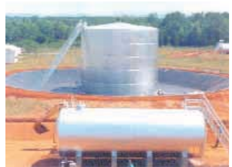
Figure 6 Liner Containing Tank and Piping
