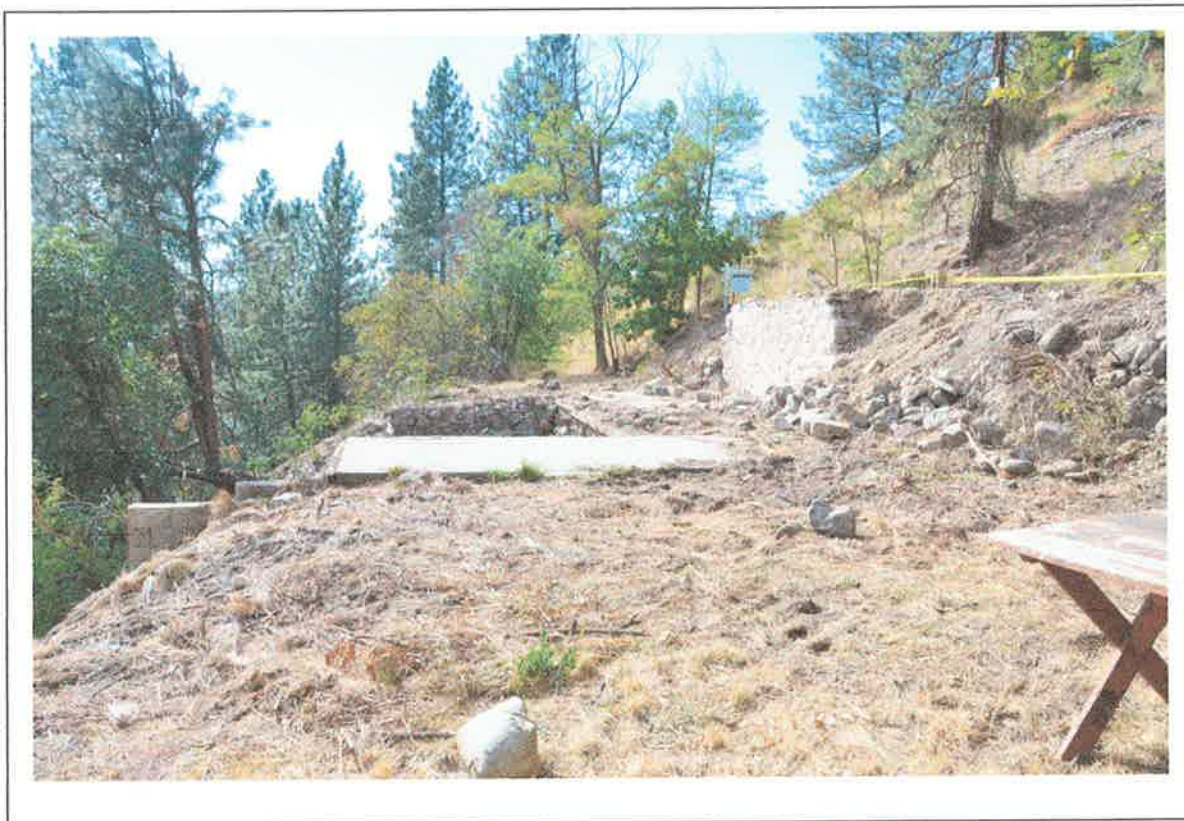
Photo 4 – View to West Across Site Showing Foundations and Slope Break on South
