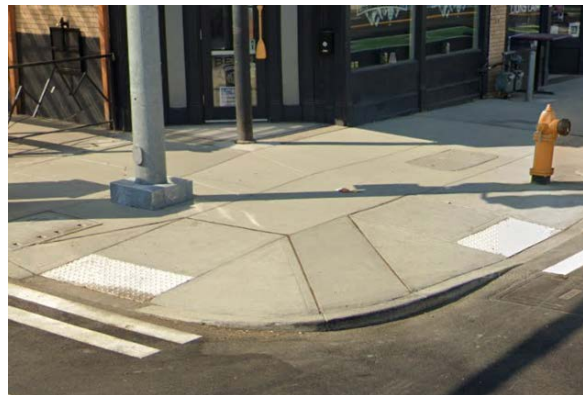
Image 4: Dual curb ramps are the standard for new construction in the City's design guidelines.
