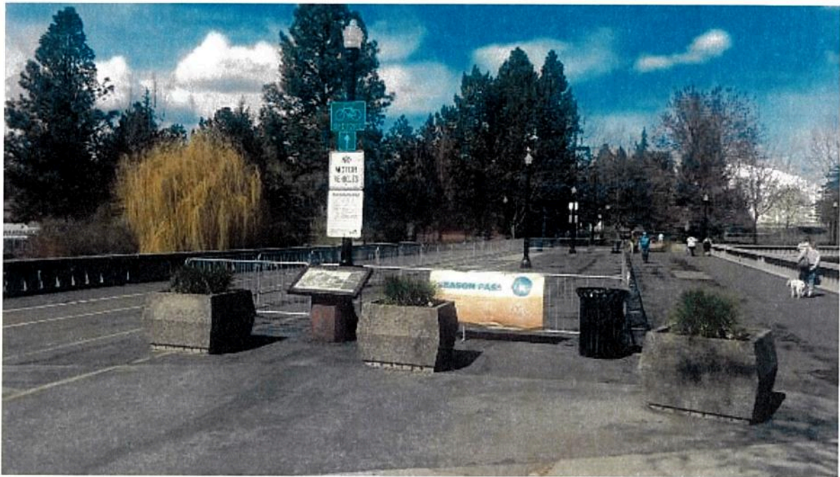
Photo 4: At south end of the Howard Street South Channel Bridge looking north. Shows barricades in the center of the bridge restricting passage and load weight because of bridge's poor structural conditions.
