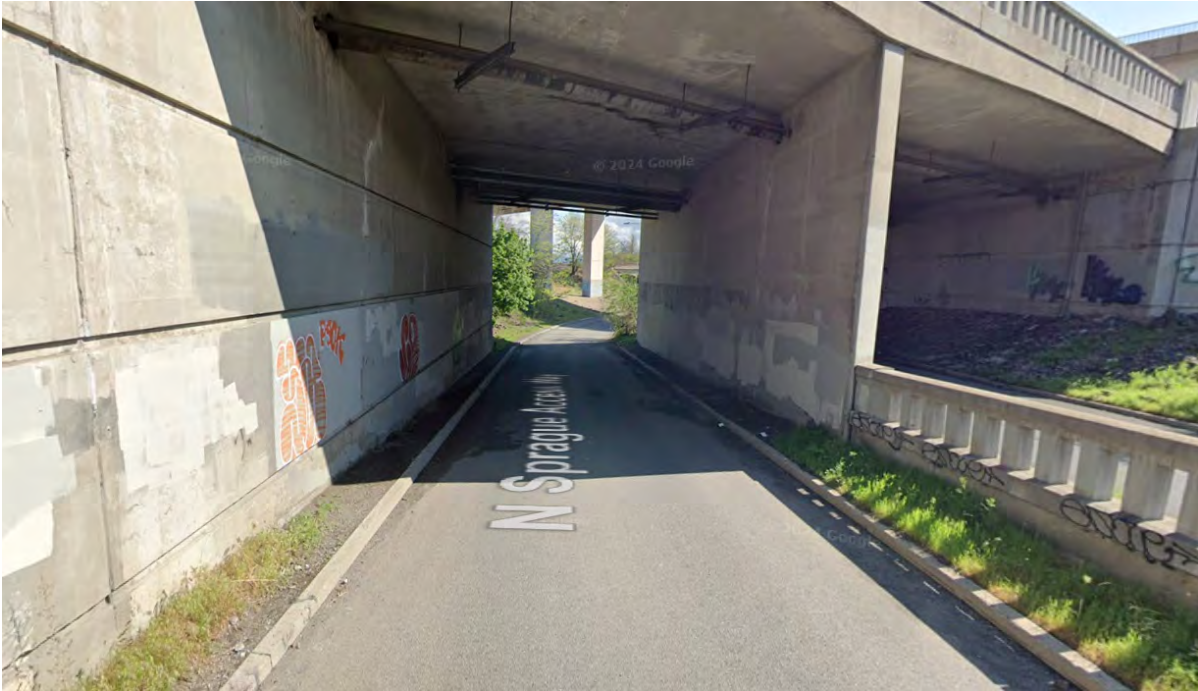
Figure 21: N Sprague Access Way, at Sprague Ave Overpass, facing North (from Google Street View)
