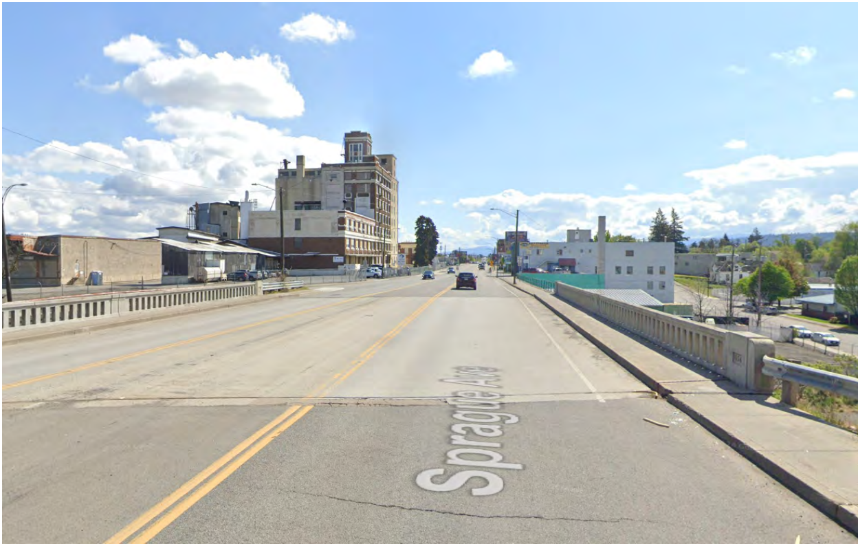
Figure 12: Sprague Ave, east of SR-290, at overpass of Erie St, looking East (from Google Street View)
