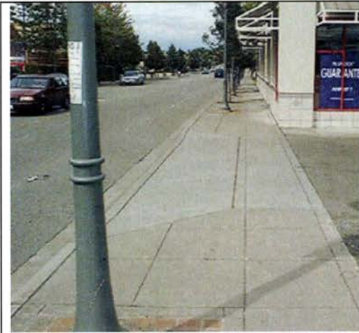
Figure 17C.123.050-E: Curb cuts and driveways may not interrupt sidewalk material and pattern requirements. Ramps may not encroach on Clear Pedestrian Zones.
