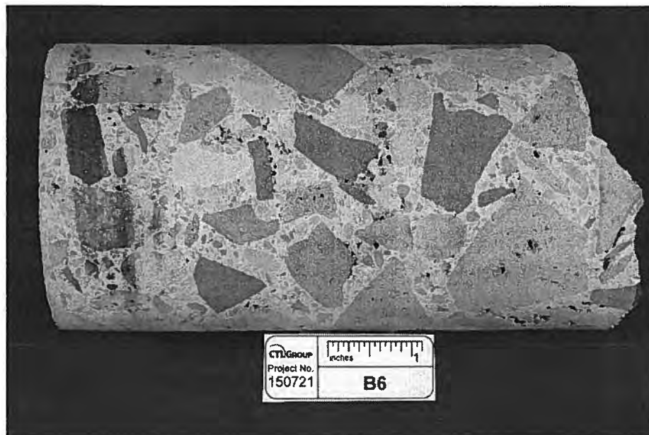
Fig. 2 Side view of Core B6 as received. Exterior surface at left.
