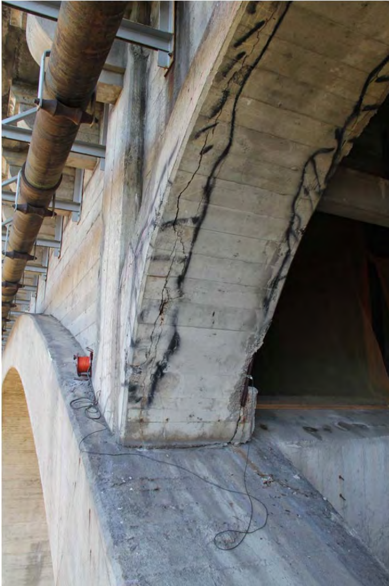
Photograph 3 - North Spandrel Wall Column Delaminations on Intermediate Arch Corners
