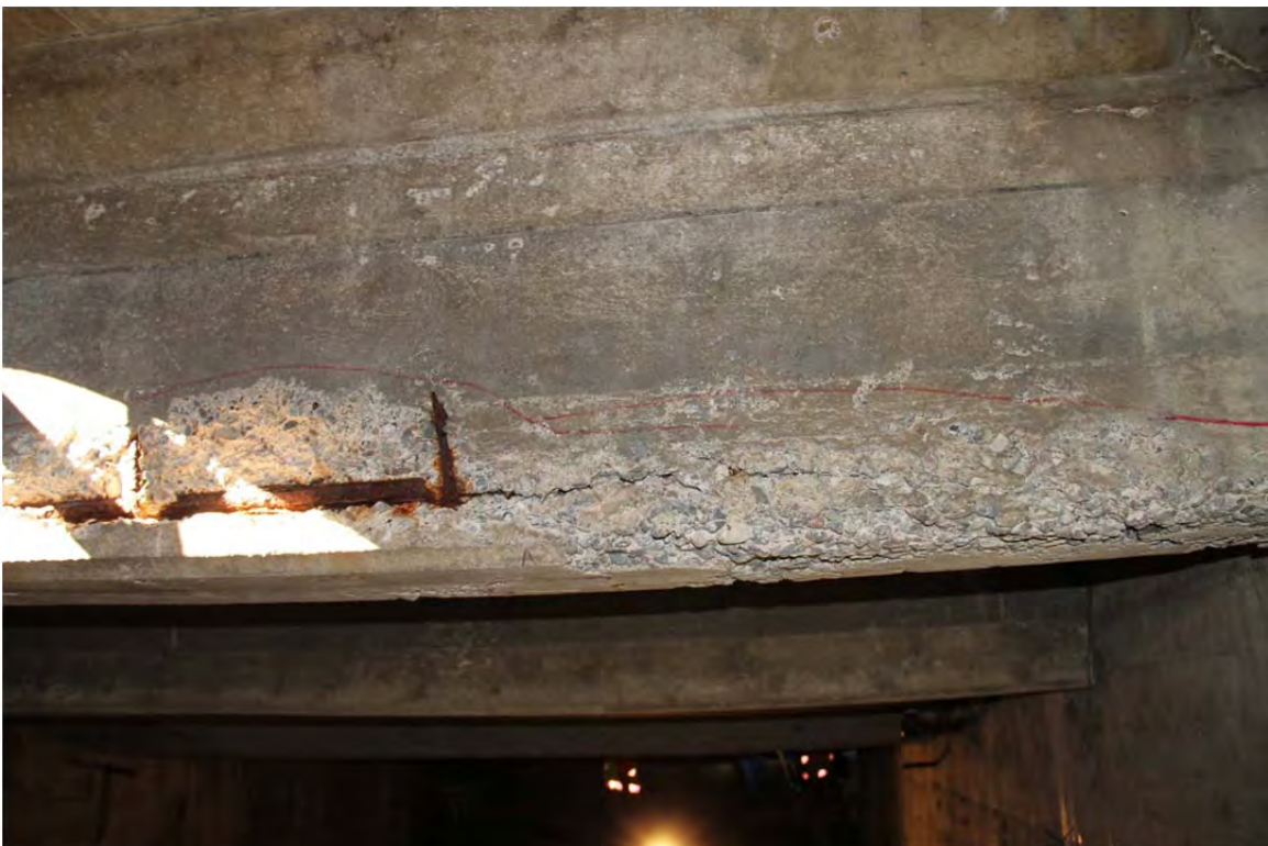
Photograph 6 - Corrosion and Delamination at honeycombed concrete
