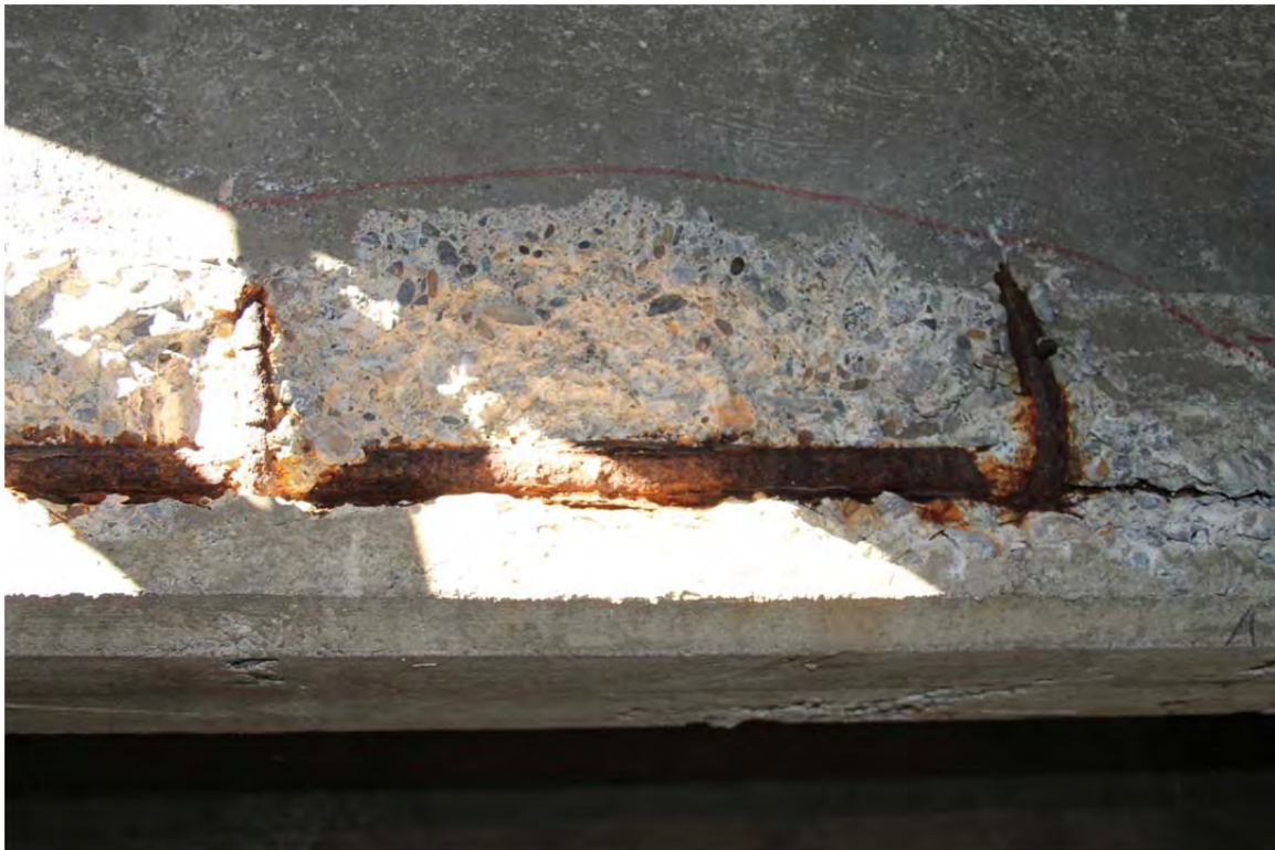
Photograph 4 - Pier 2 Interior Floor Beam Corrosion
