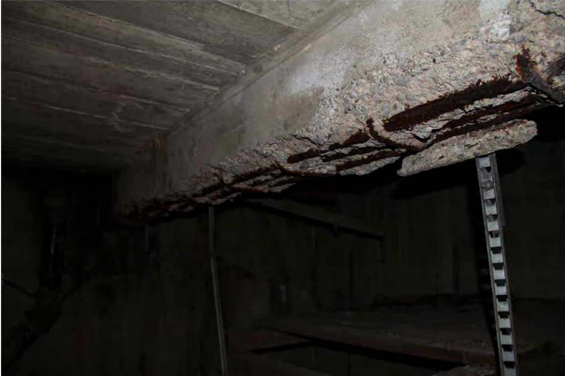
Photograph 7 - Delamination on bottom of floor beam
