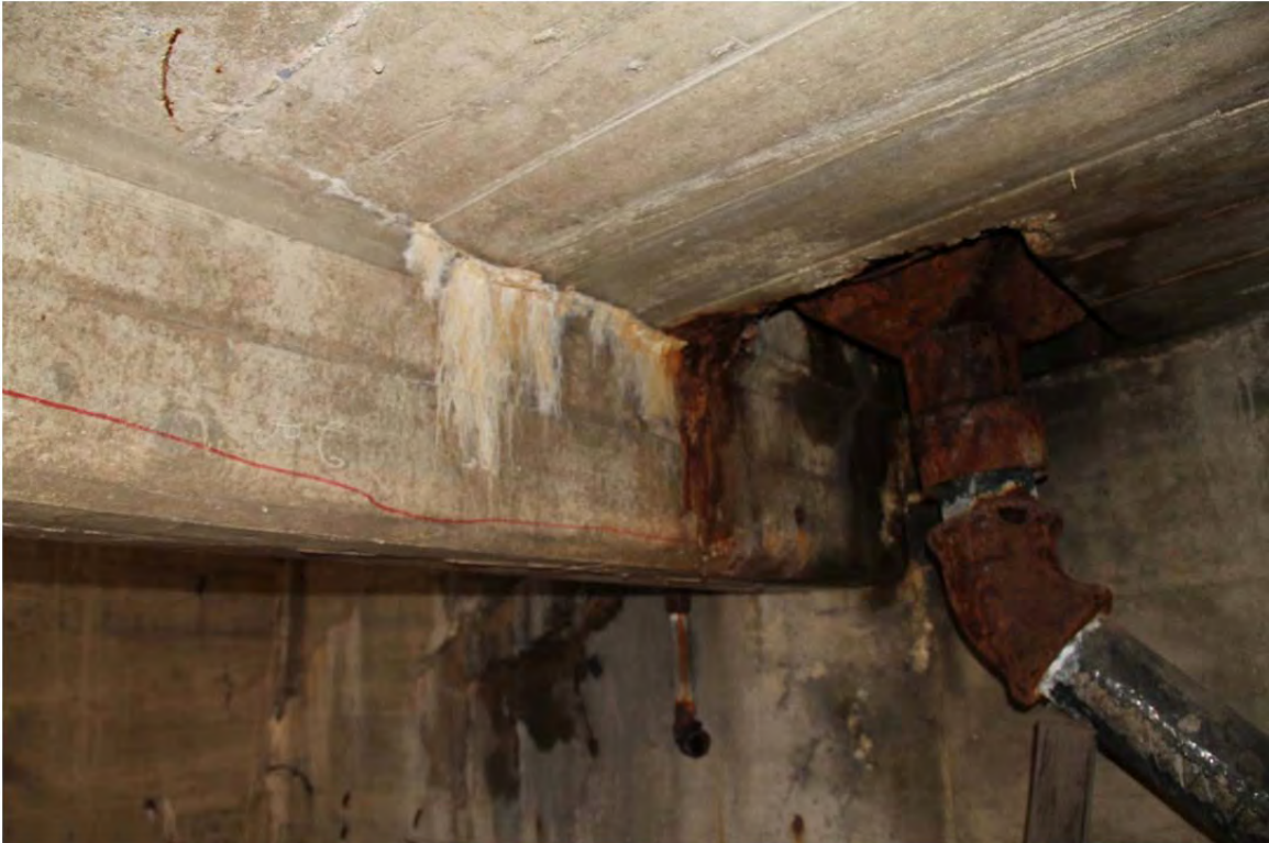
Photograph 5 - Corrosion in Pier 2 at drain pipe leakage
