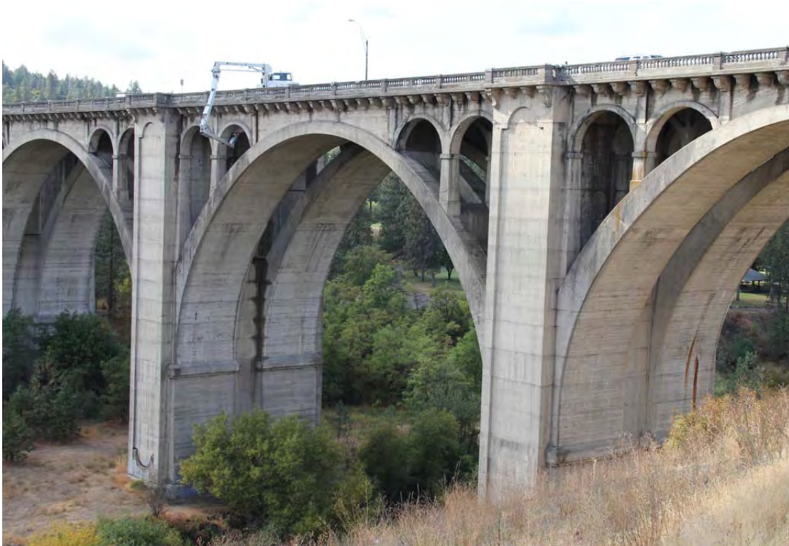
Photograph 1 –Water runoff areas between spandrel wall column and pier.
