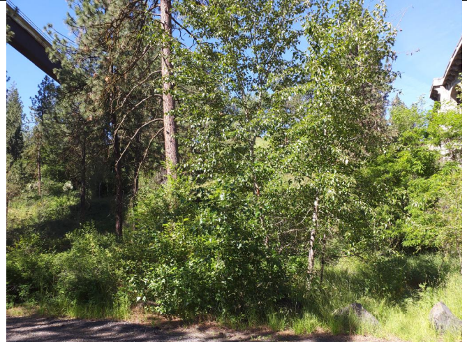
Photo 4: Potential seep area at toe of slope.
