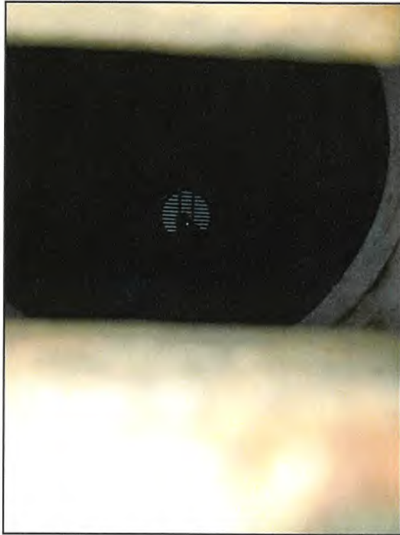
PHOTO 5: TP-1 STANDING WATER WITHIN DRYWELL
