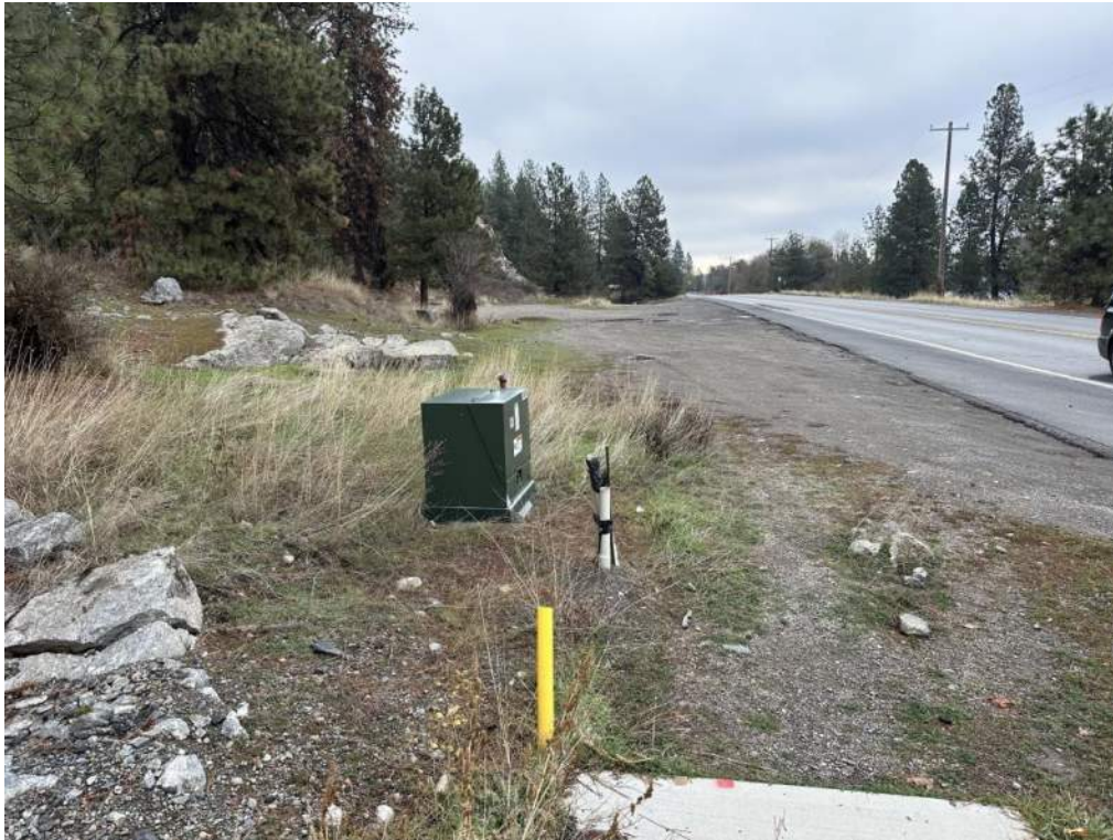
Photo 11. Pictured are the existing utilities on the western edge of John H. Shields Park, facing east. Utilities will tie into this existing infrastructure.
