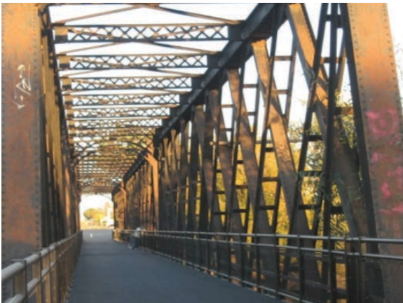
The Iron Bridge, as it is colloquially known, provides an ideal pedestrian crossing over the Spokane River.
