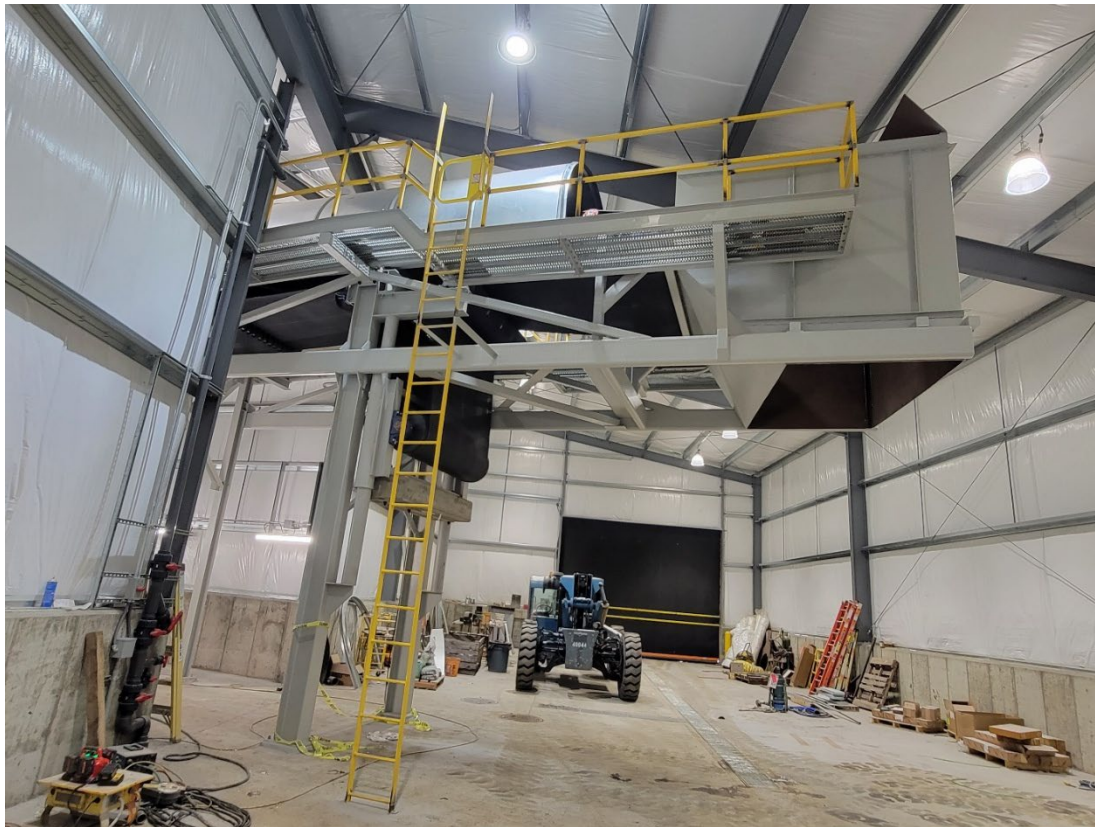
Outlet/Drop Chute for the New Ash Conveyor. KCS Designed, Fabricated and Installed (Completed in 2022)
