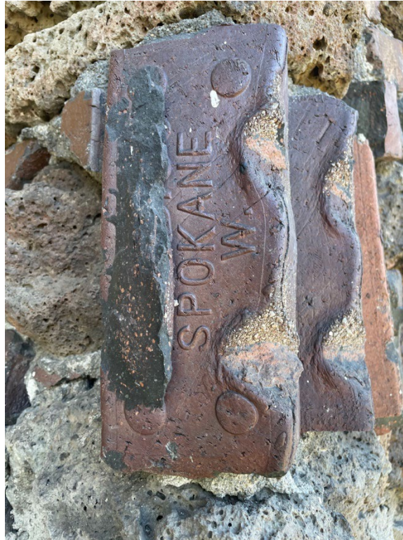
Figure 24: Vertically oriented, misshapen brick in rubblemix column
