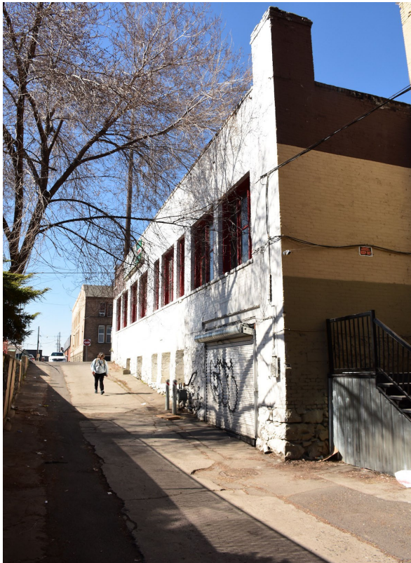
The rear southeast corner of the building where it extends behind the neighboring building to the east.
