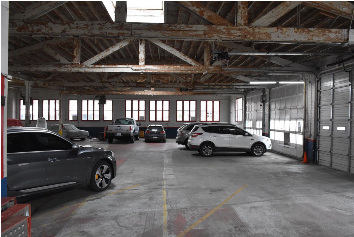
15. Main floor - west bay cochere entry, looking south at roll-up garage door
