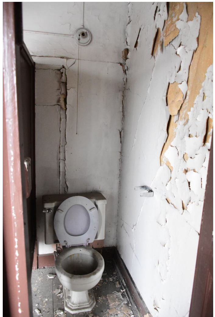
#31. Third floor restroom-toilet, northwest corner
