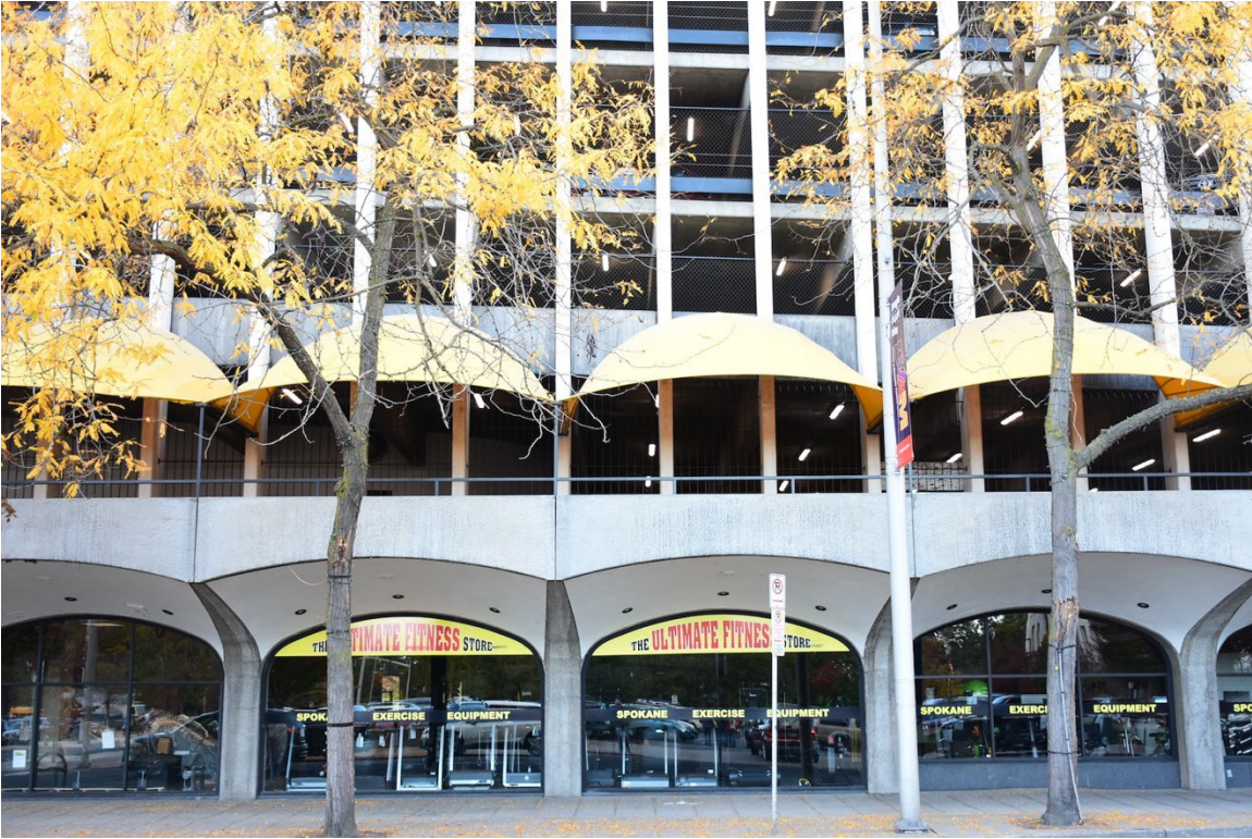
8. North facade, east of ramp, looking south at storefront and skywalk level (floor 2) (10/2023)
