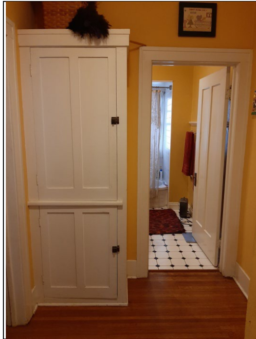
Photo 14 A 2023 photograph of the linen closet and the interior hall at the first floor
