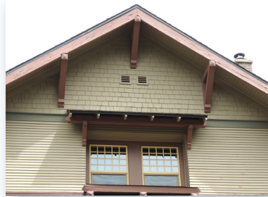
Brackets on the house at 1010 W Thirteenth
