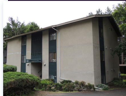
Vertical Plane Breaks at 909 W Thirteenth
