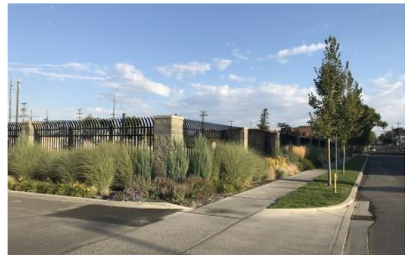
Avista Cedar Street Substation | Spokane (2015)
