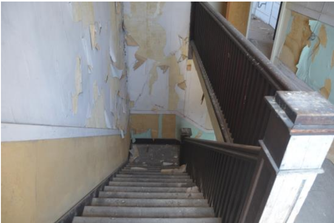
25. Stairs in Southwest Corner, Looking Down From 5th Floor to 4th Floor
