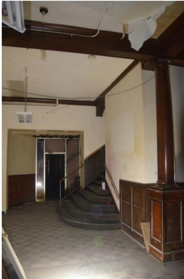
15. Lobby, Northwest Corner, Door to Retail Bays, Stairs to 2nd Floor, Looking North
