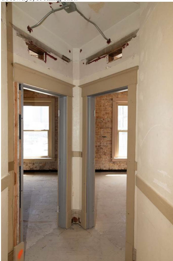
Photo 0031. Second floor, typical branch hallway showing the angled vestibule at the unit doorways, looking east.
