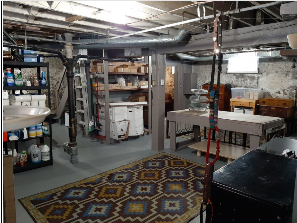
Photo 19 2024 photograph of unfinished basement
