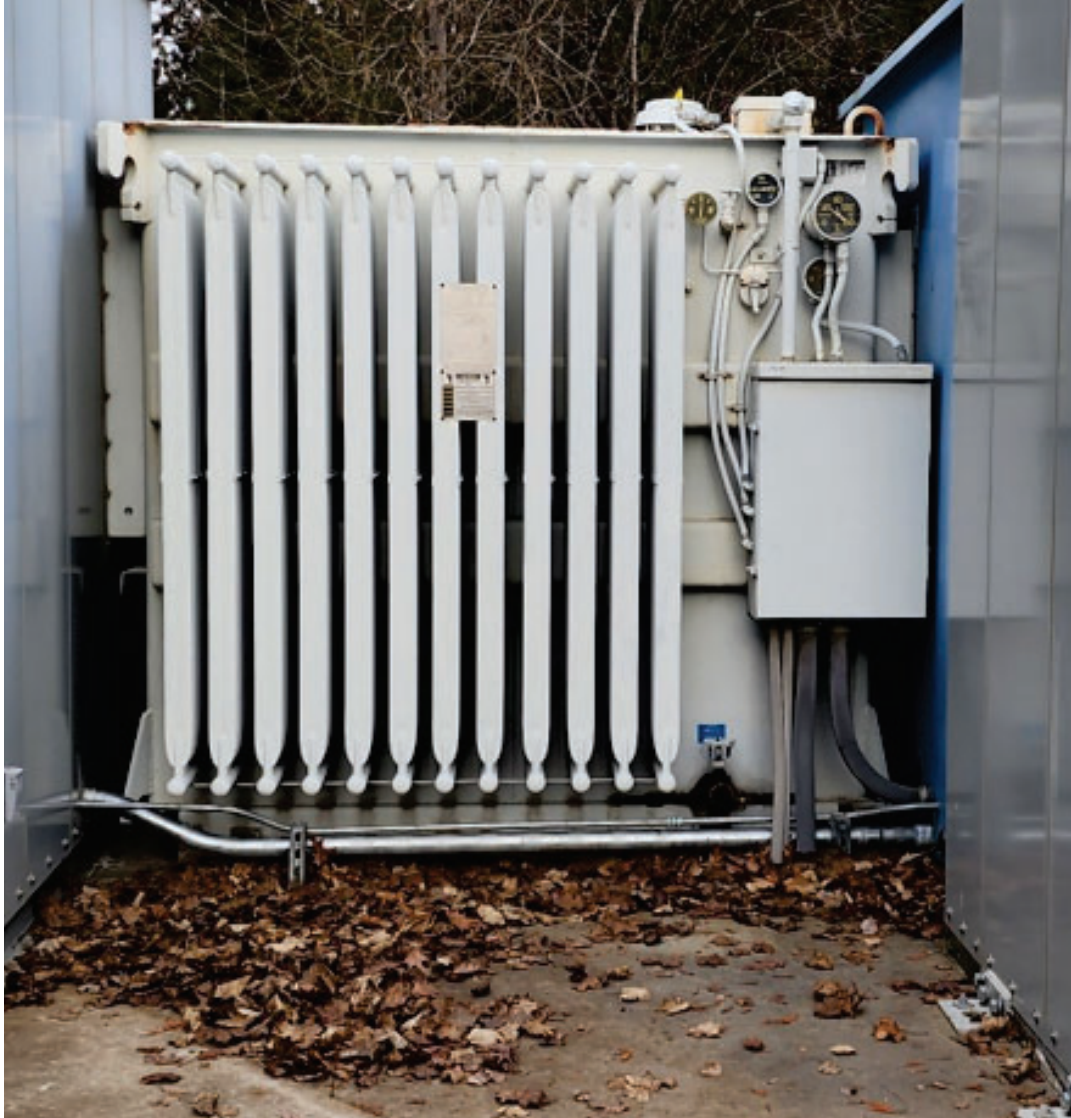
Switchyard 2 GSU transformer
