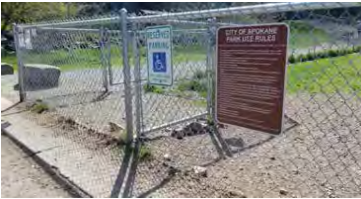
Image B.5 - The corral at the small dog park area for Highbridge Park. The gravel surface has eroded leaving large gaps under the fence small dogs can escape through. There is no paved access to the gates.
