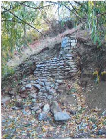
Manhole sandbagged in 2012 due to erosion 2012.
