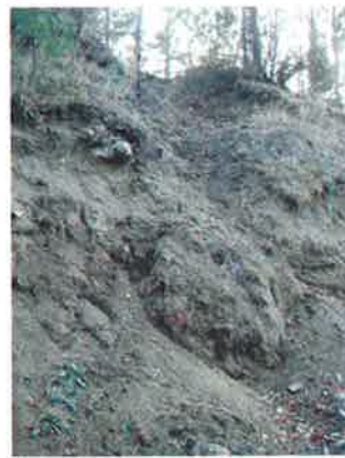
Eroded path from below.
