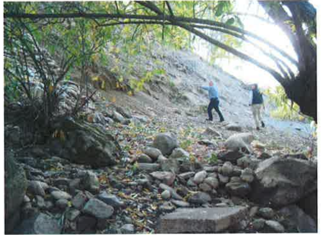
View from manhole downstream showing sandy eroded riverbank.
