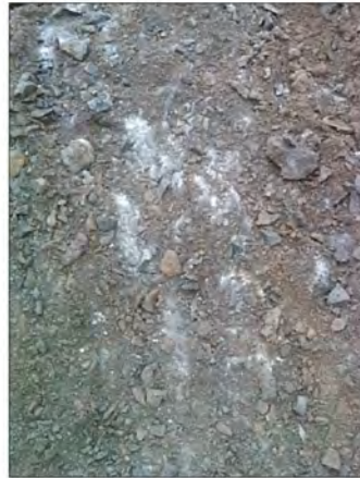
Photograph 5 – View of basalt rock in TP-6 excavation base (looking down at test pit bottom).
