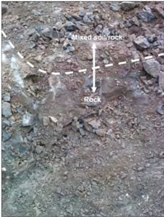
Photograph 4 – View of TP-6 sidewall showing mixed soil and rock overlying fractured basalt rock.
