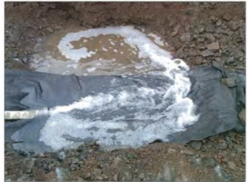
Photograph 3 – View of water discharge methods for large-scale flood test performed in TP-6.
