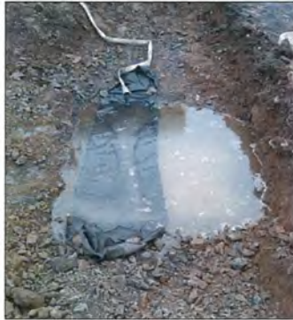
Photograph 2 – View of large-scale flood test area performed in TP-6 (overflow infiltration area).
